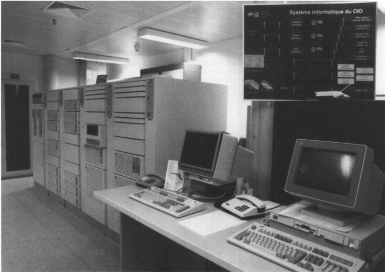
The "machine room" in the basement of Olympic House.
